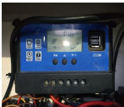
Gambar 3. 3 Solar Charge Cotroller
